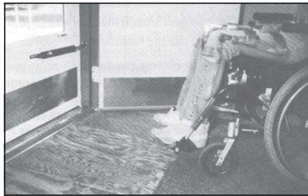
Figure 4. Installing kick panels on both sides of doors protects them from wheelchair damage.
